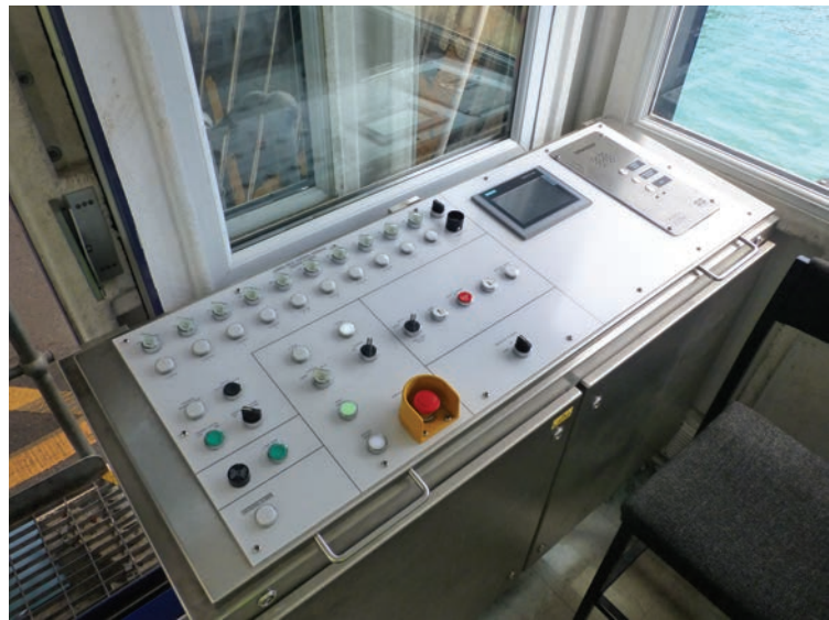
Control station | Berth 6 linkspan, Dover Port
